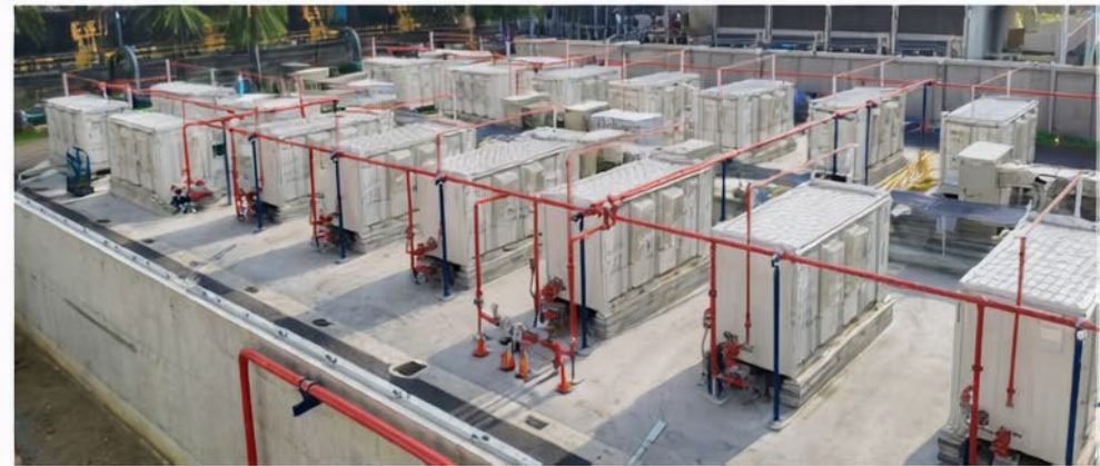
Xingang Energy Storage Facility
